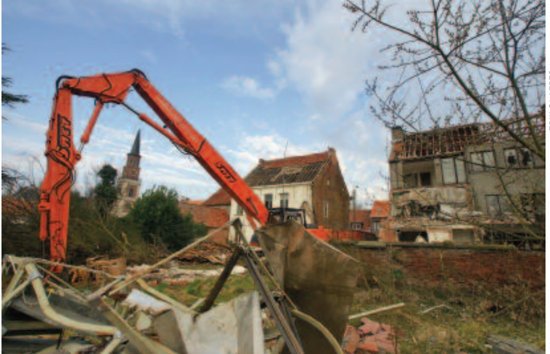
Demolition in Doel. The Belgian government is unable or unwilling to prevent the destruction of the entire village, including several listed historic buildings, even though the economic basis for its eradication vanished with the worldwide recession
